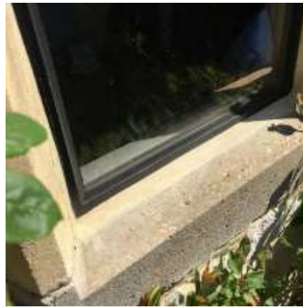
Detail of good practice: colour and scale to fit at Spring Cottage replacing the original metal casement and maintaining light levels within the cottage. Original fixings were reinstated.
